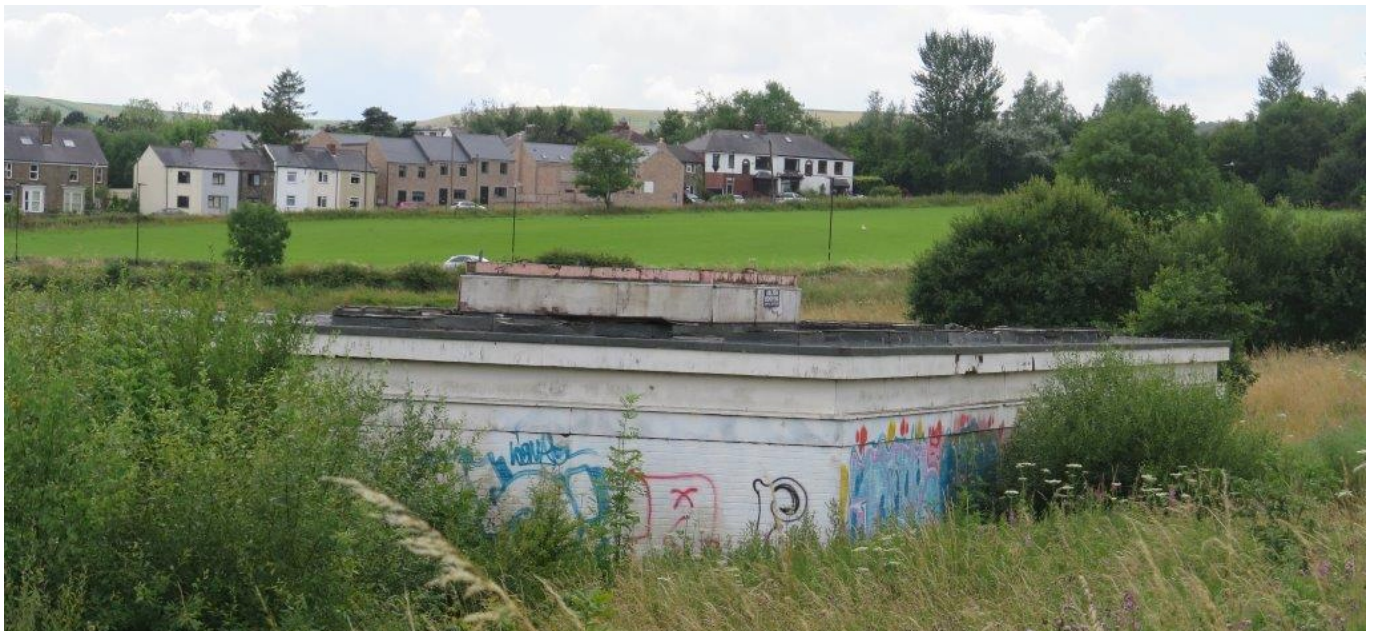
Derelict Sports Pavilion off Cross Lane
